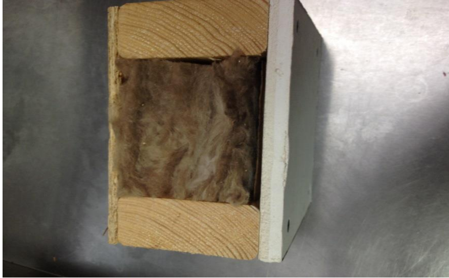
Figure 2.5 Picture of the inside of the residential building wall showing the wood studs and batt insulation.
